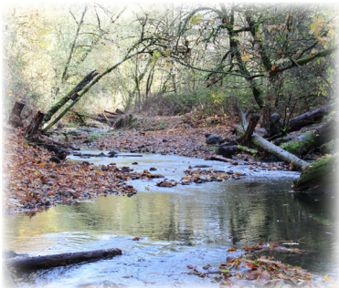
Over 20 large wood structures along with boulders were placed to restore fish and wildlife habitat in Rock Creek
