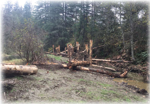
Large wood structures placed to restore fish and wildlife habitat in Clear Creek.
